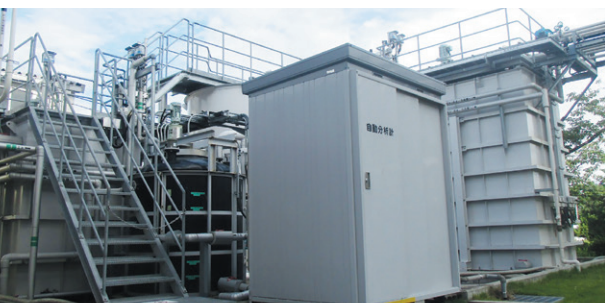
Wastewater processing equipment
